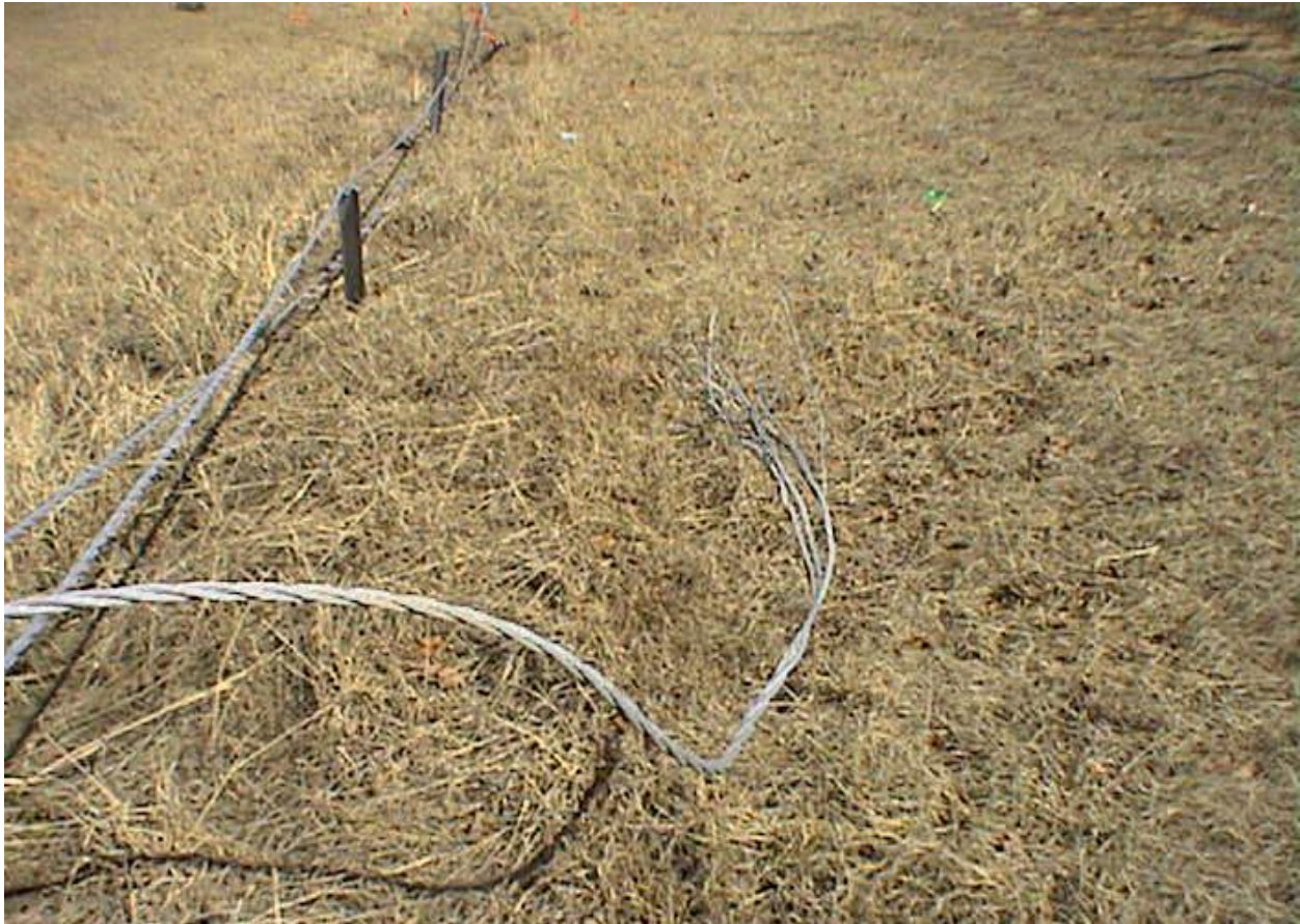
Figure 67. High-Tension Splice Tearout Penetration
